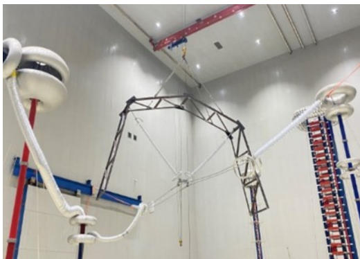
RIV and Visual Corona Test of 345kV suspension string in SHEMAR's Electrical Test Hall
