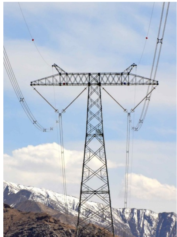
± 400kV DC Qinghai-Tibet Project
