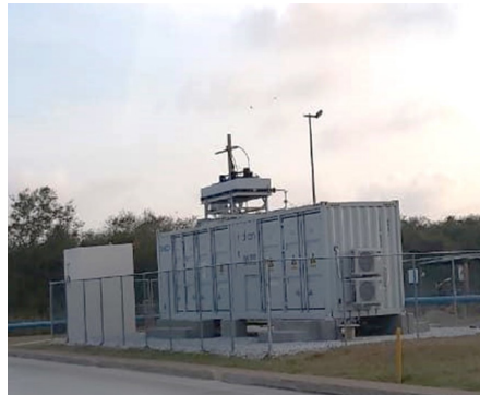
Galvanized steel 4 MVAR STATCOM
