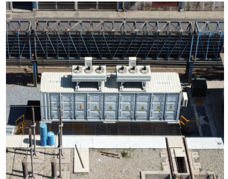
Rolling mill 15 MVAR STATCOM
