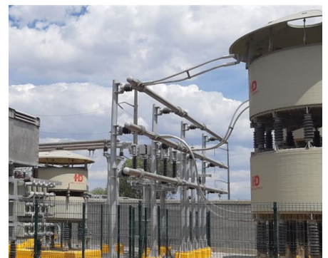
Steel (EAF) 110 MVAR SVC
