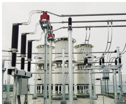
Steel (EAF) 75 MVAR SVC
